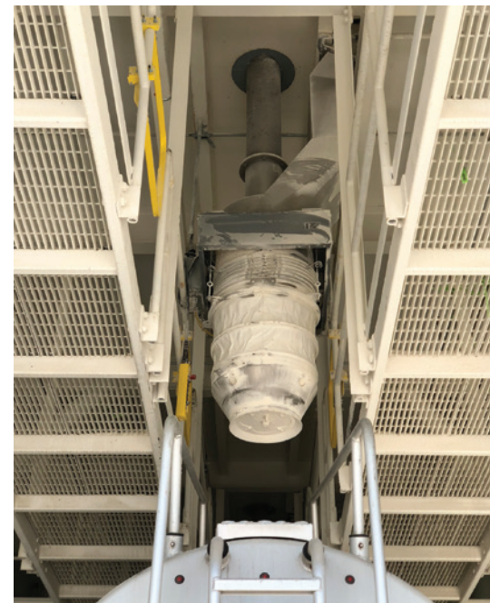
Telescoping Loadout Spout & Exhaust Duct
